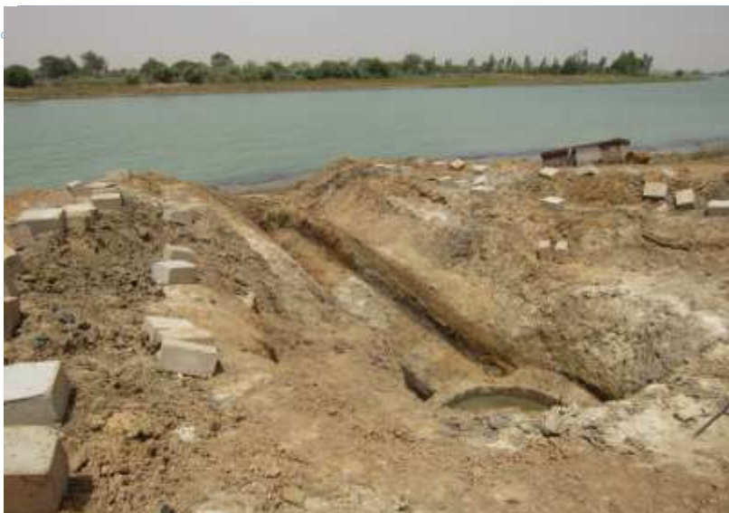
Intake channel for the pump and sump
