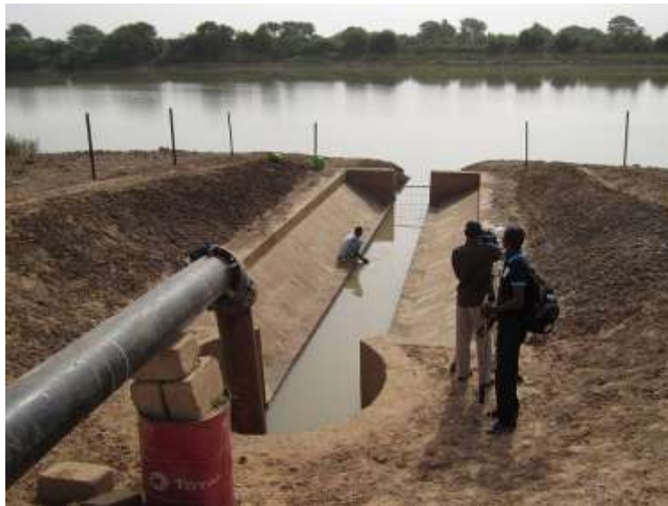
Intake channel for the pump and sump
