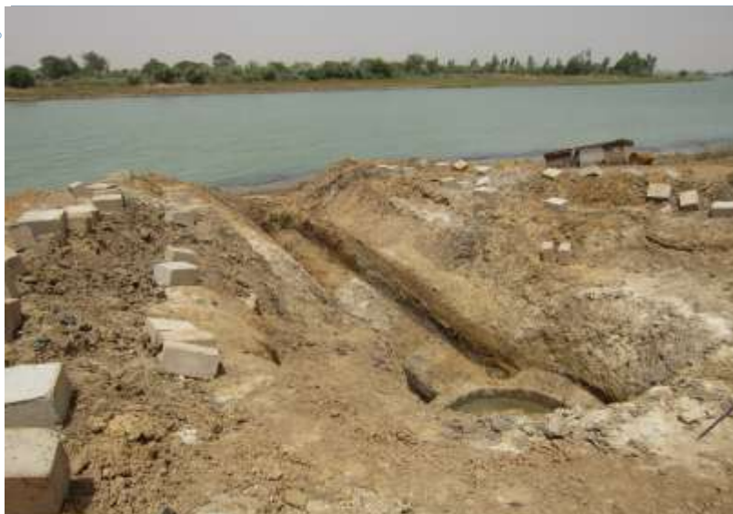
Intake canal of the pump and suction pit
