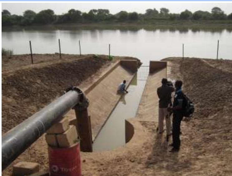
Intake canal of the pump and suction pit
